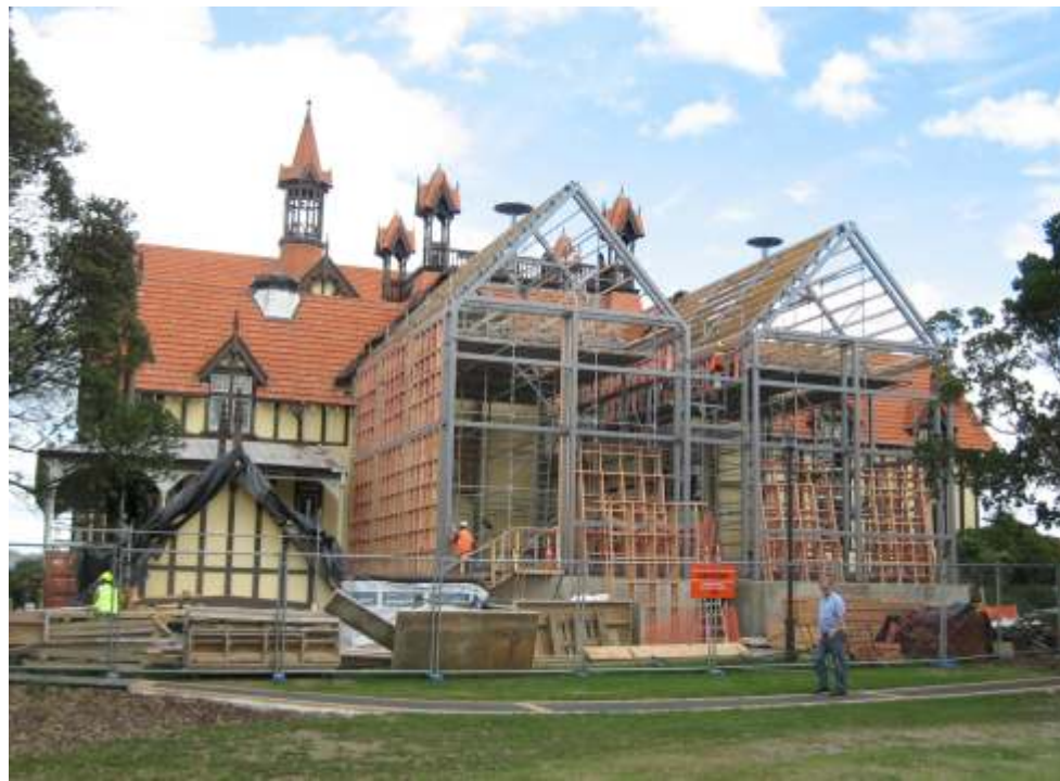
The detached pediment gable, which can be seen sitting to the left of the new wing, will be reattached when the exterior nears completion.
